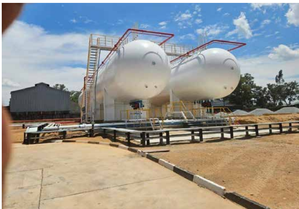
NOIC LPG Storage Depot in Ruwa
